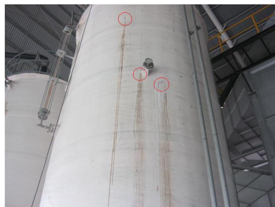
Gambar 2. Kebocoran tangki GFRP sludge tank
