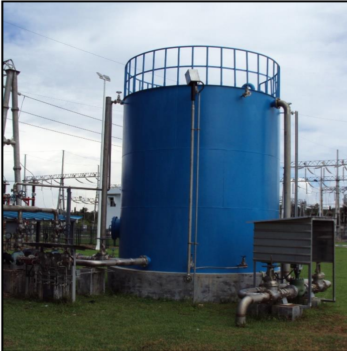
Figure 6. Condensate Storage tank
