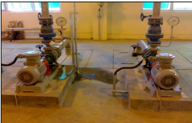
Figure 1. Desalting water pump.
