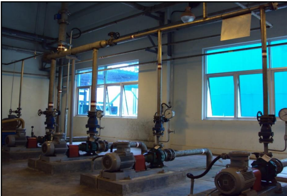
Figure 4. Tapping at desalting water pump and regeneration pump after redesign
