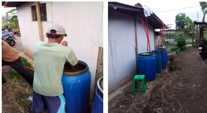
Gambar 5. Instalasi biogas drum
