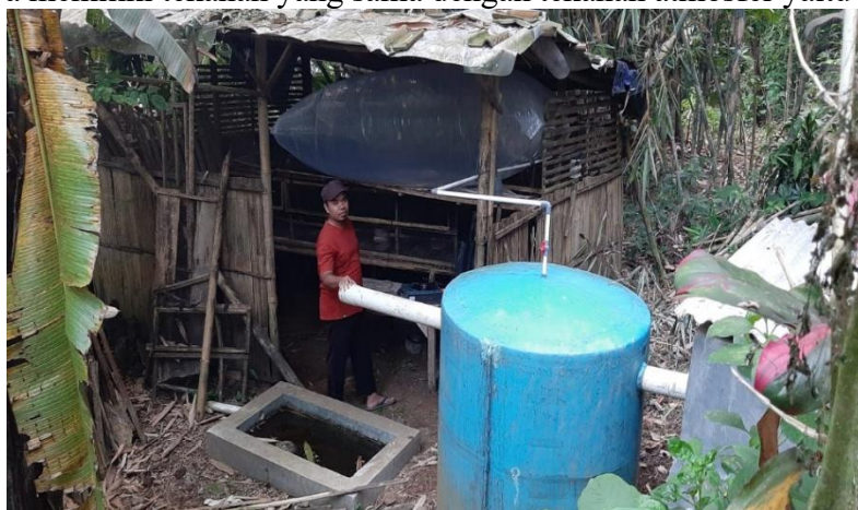
Gambar 6. Instalasi biogas fiber tanam
